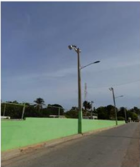
Light system of baseball stadium in Pedernales
