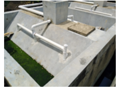
Figure 6: UASB status, August 2021. Photo: ©GIZ/ PROAMSA
