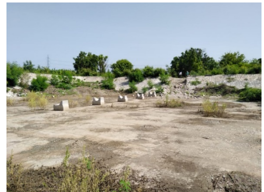
Figure 3: Status of the facultative lagoon in August 2021. Photo: ©GIZ/PROAMSA
