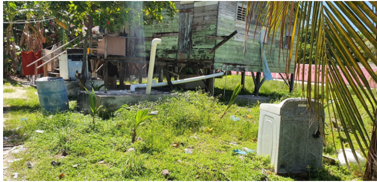
Figure 1: Above-ground septic tank in Caye Caulker, South Region. Photo: ©GIZ/AKUT
