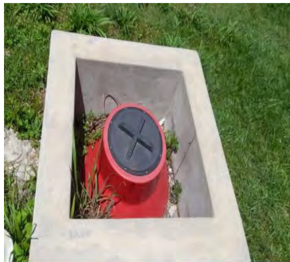
Figure 10: Precast plastic ST (Source: Jodian/Org./2022).
