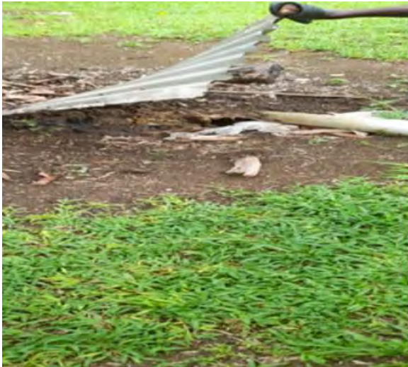
Figure 7: Broken sewer pipe leading to soak pit (Source: Jodian/Org./2022).
