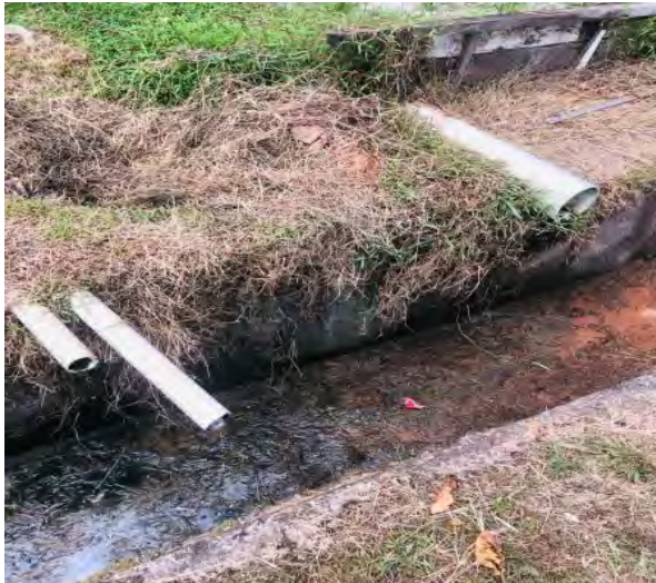
Figure 4: Pipe connected to Open Drain (Source: Rabicia/EPA./2022).
