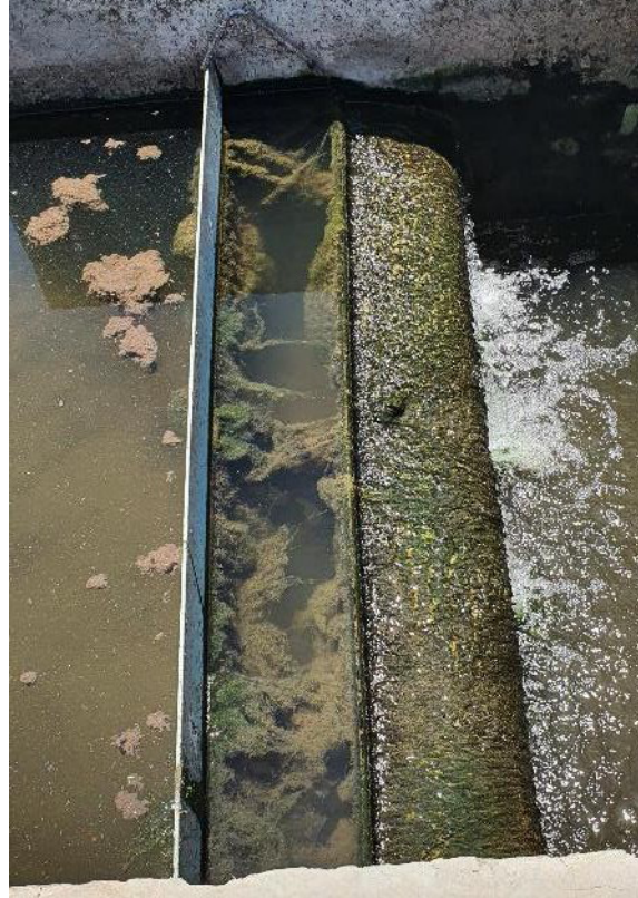
Figure 8 - Innswood – chlorination basin discharge
