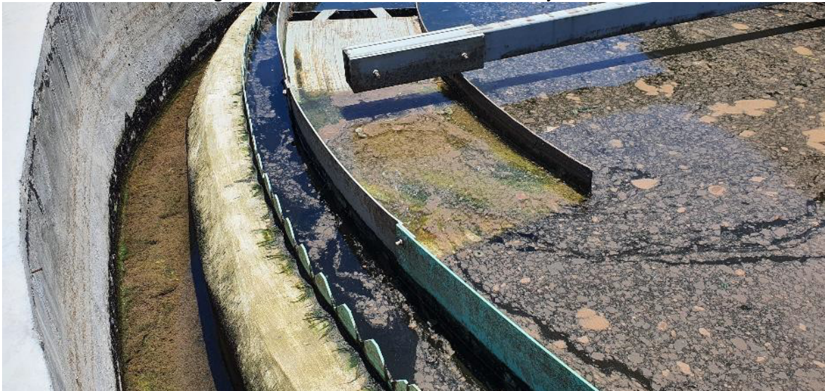
Figure 9 - Innswood – overloaded secondary clarifier
