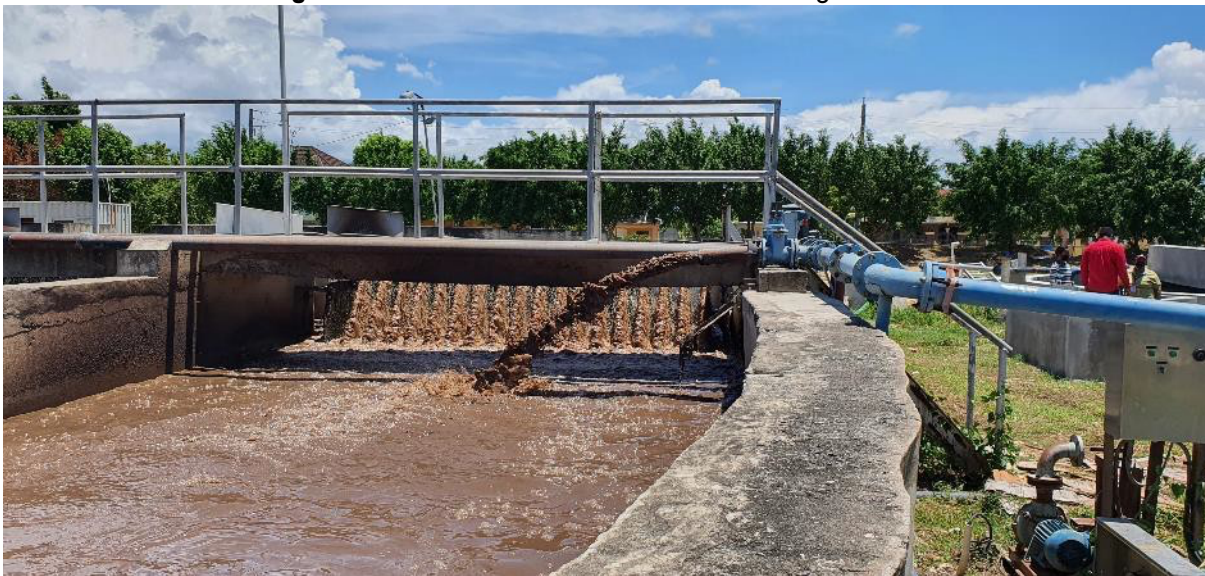
Figure 7 - Innswood – oxidation ditch with sludge return
