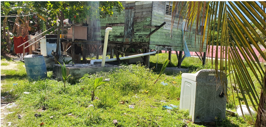
Figure 2: Septic Tank in South Caye Caulker
