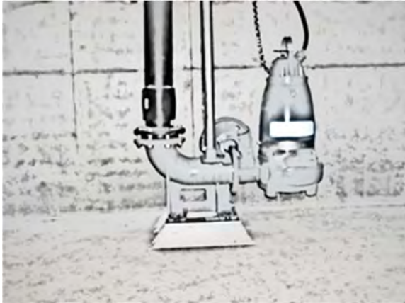
Figure 19: Pumping station with submersible cutter pump
